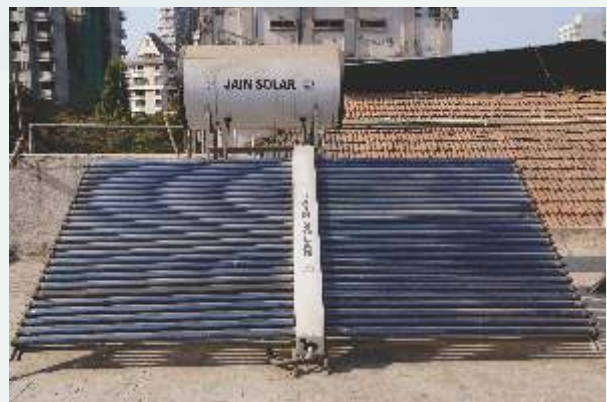
Fig. 15.6 Rooftop Solar water heater
