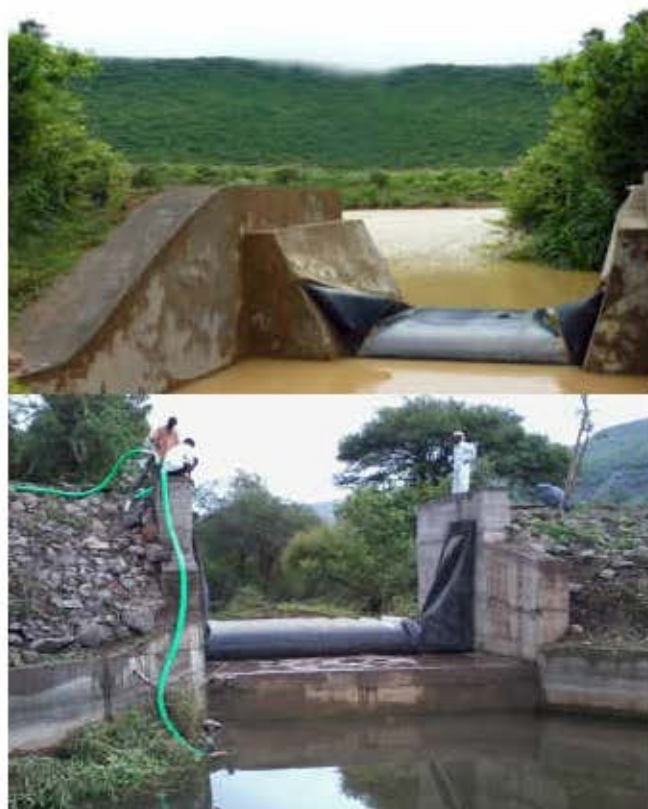
Fig. 3.1 Demonstration of inflation and deflation of the ICAR flexi check dam at Kanse village, Ambegaon Taluka, Pune district
