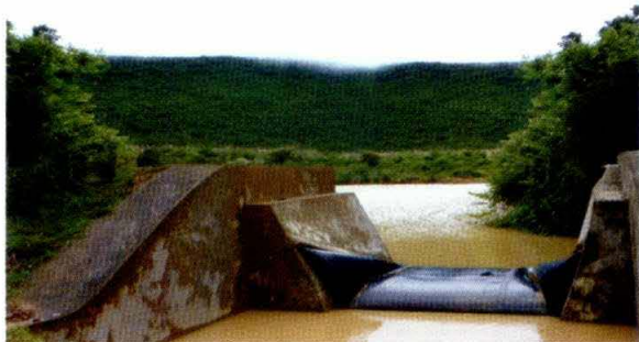
Fig. 8. Rubber Dam installed at Badaphokaria, Khurda District, Odisha
