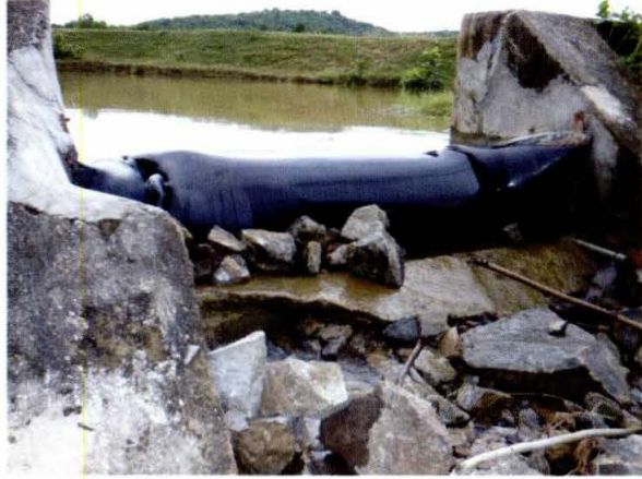
Fig. 6. Rubber check dam installed at the experimental field of Directorate of Water Management (DWM), Mandhasal, Odisha
