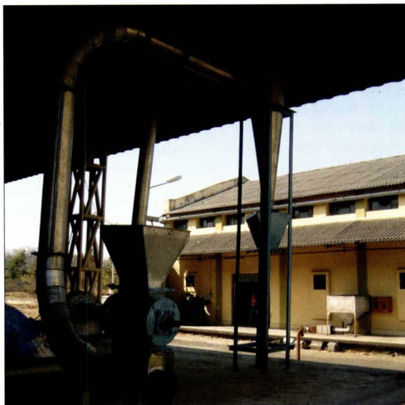
Fig.2 : A Fabricated System of Cyclones at GTC, Nagpur
