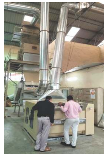
Fig 2.1.2: Air Jet Cleaning System installed at GTC Nagpur
