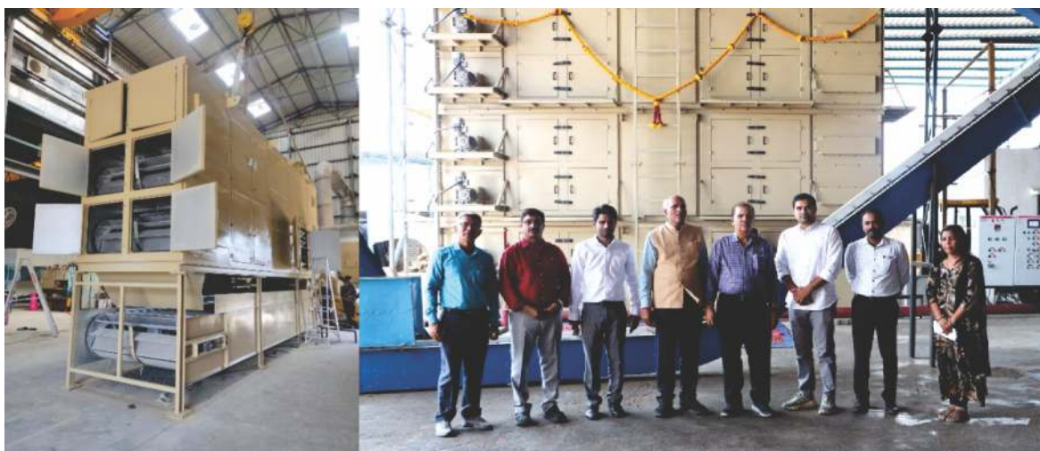
Fig.2.1.1 Energy efficient continuous flow Cottonseed dryer (installed in the ginning factory)
