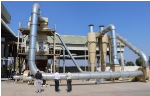
Fig. 2.4 Seed cotton contamination cleaner installed in ginning industry
